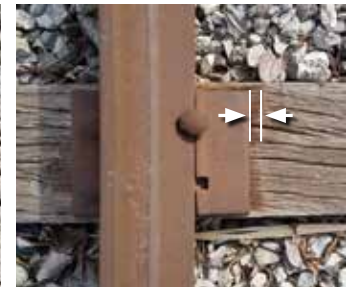
Tie plates rubbing ties
