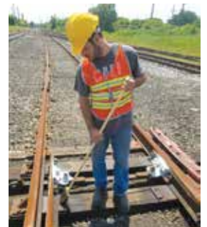
Track Switch Maintenance
